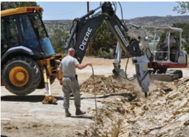
Engineers from the 184th Intelligence Wing Civil Engineering Squadron dig a trench for a new sewer and water system for an existing house during their annual training. The work was performed in conjunction with the Southwest Indian Foundation.
