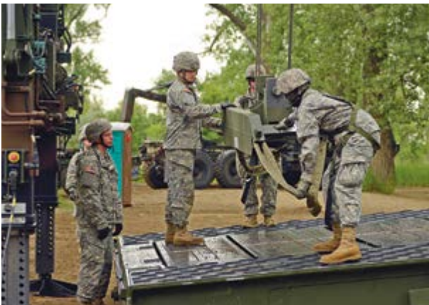
Soldiers with the North Dakota National Guard's 957th Engineer Company (Multi-Role Bridge) assemble a dry support bridge at Kimball Bottoms, south of Bismarck, June 18, 2014.
