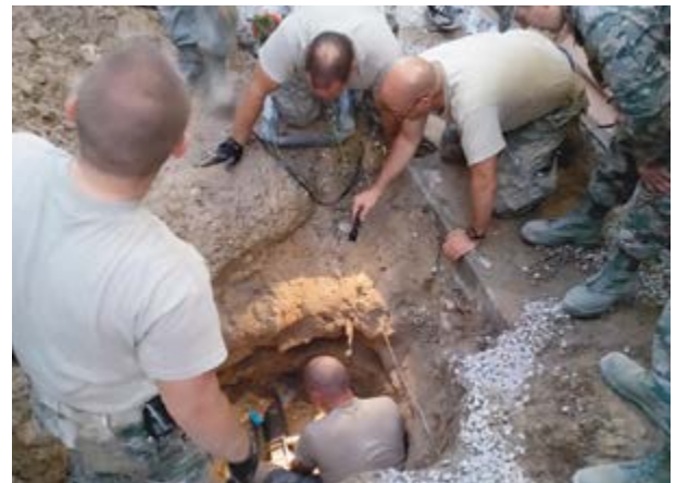
Senior Airman Loal Lee, 151st CES, Utah Air National Guard, repairs a water leak at a deployed location in support of Operation Enduring Freedom, Aug. 26, 2014.
