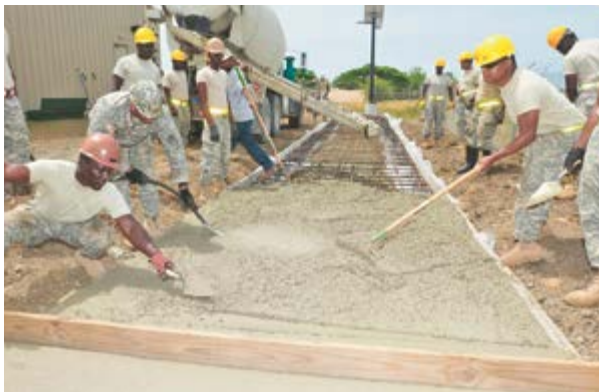
Members of the Detachment 1, 1011th Engineering Company distribute and smooth poured concrete during a construction project at the Estate Bethlehem Training Site on St. Croix, July 19. The 1011th EN Det. conducted annual training for two weeks on St. Croix, during that time numerous projects were completed, including the concrete base for a set of bleachers.
