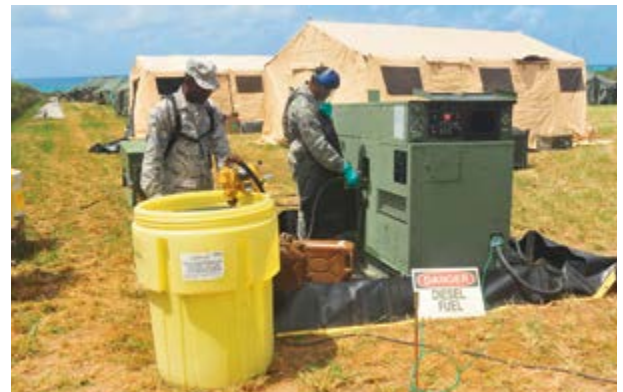
Senior Airman Anthony Harley, a power production journeyman with the 285th Civil Engineer Squadron, pumps fuel into a MEP806 diesel generator while Airman 1st Class Moses President, a member of structure, monitors the fuel source, June 7. The Virgin Islands National Guard had a large contingent of Soldiers and Airmen camped out at Camp Phoenix on St. Croix's South Shore during Operation Forward Guardian II, a disaster-relief exercise.
